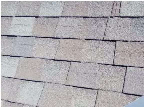
Cracks in shingles.
