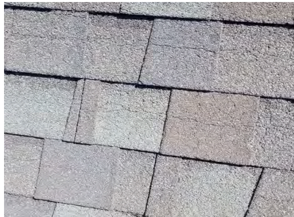
Cracks in shingles.
