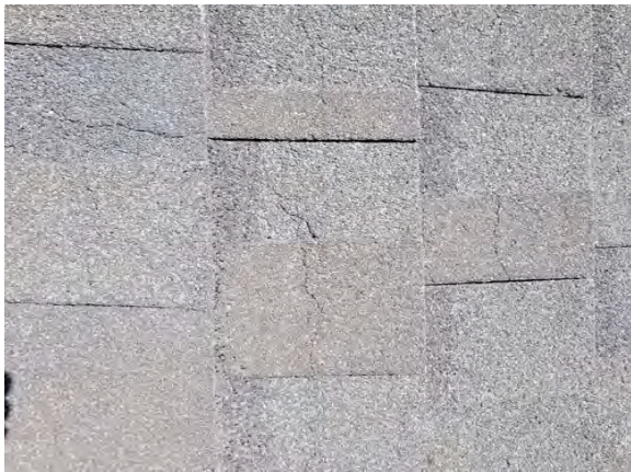
Cracks in shingles.
