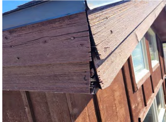
Facia on upper roof is starting split.
