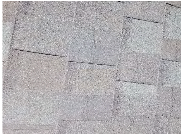
Cracks in shingles.
